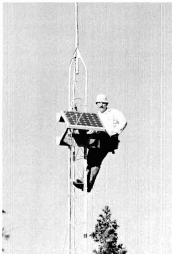
Co-author WB5RSN makes final angle adjustments to solar array that powers the 19-79 repeater on Redondo Peak, New Mexico (3433 meters, 11,254 feet). The array is mounted at 17 meters (55 feet) to prevent shading from nearby trees.
